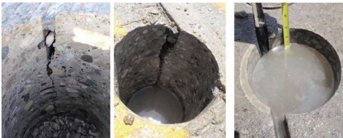
Examples of subbase drainage at pavement core holes. Good, medium and poor drainage, from left to right, respectively.
