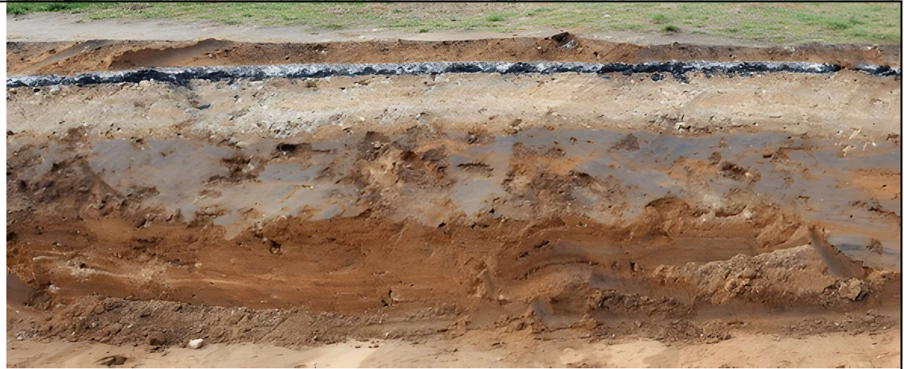
Cross-section of the pavement with layers of clay sand and asphalt. Panoramic collage from several outdoor photos
